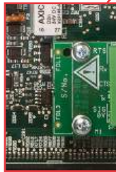
Internal view of panel
